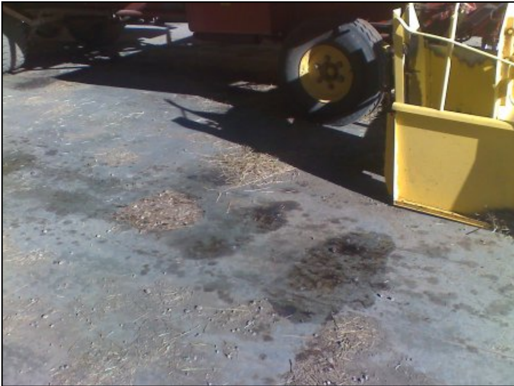
Oil stains located on the concrete slab inside the hay shed.
