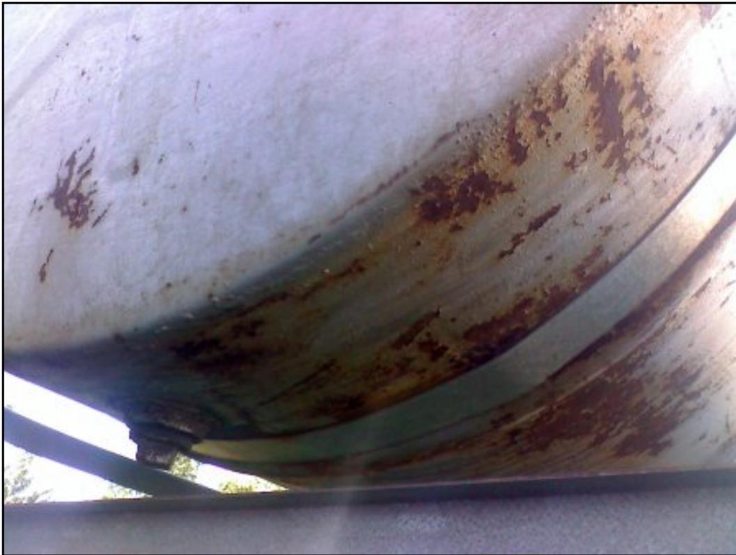
Surficial rust located on the underside of the AST.
